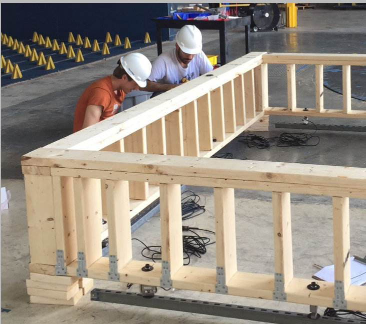
Florida International University REU students Ahmed Saleh (in white) and Walker Hood (in orange) installing the load cells for a Department of Emergency Management project. The structure would be tested under high speed wind to investigate its response under such drastic conditions.
