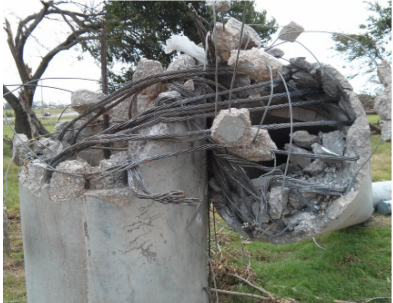
Reinforced concrete post, toppled by a tornado, May 2013, Moore, OK. (Photo: David Prevatt)
