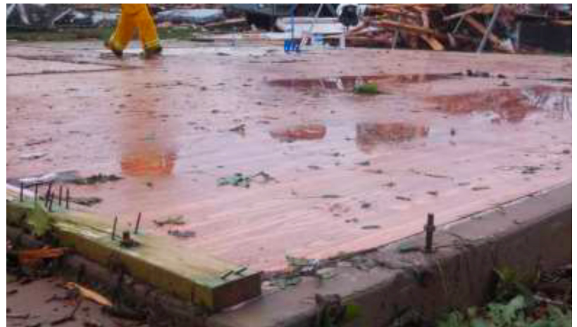
Complete destruction of home with anchor bolts just south of Hwy 377 & N. of Acton Highway in Granbury, TX. Although anchor bolts were used, the use of small washers reduced the impact of this reinforcement. Further, the lack of metal ties connecting the studs to the sill plate resulted in a weak link in the vertical load path from the studs to the sill plate. (Image: NOAA Southern Regional Headquarters)
