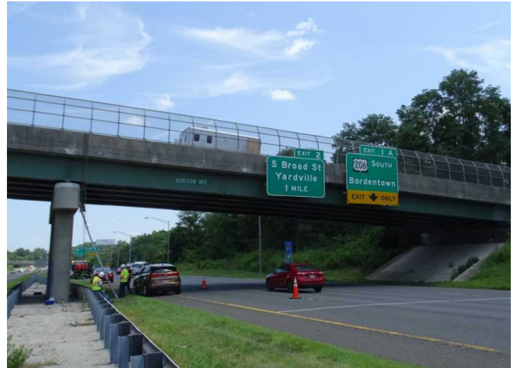
A side view of the Hobson Avenue Bridge over Interstate 195 in Hamilton Township, New Jersey.
