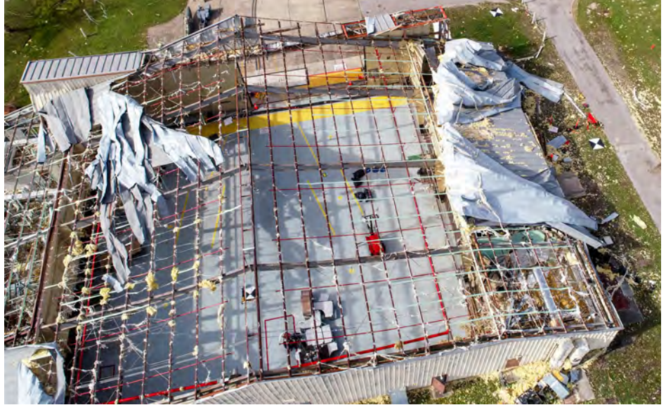
Captured by a RAPID drone, an aerial photograph shows wind damage on a large-scale industrial building following Hurricane Michael.
