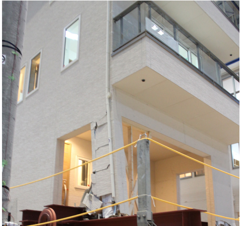
Structural and non-structural damage to a wood-frame structure. (Photo: Maria Koliou)
