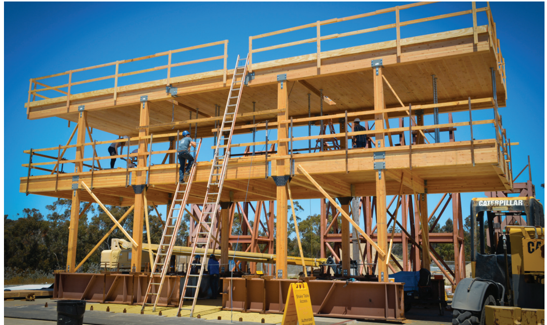
Building under construction at UCSD. (Photo: UC San Diego Jacobs School of Engineering)
