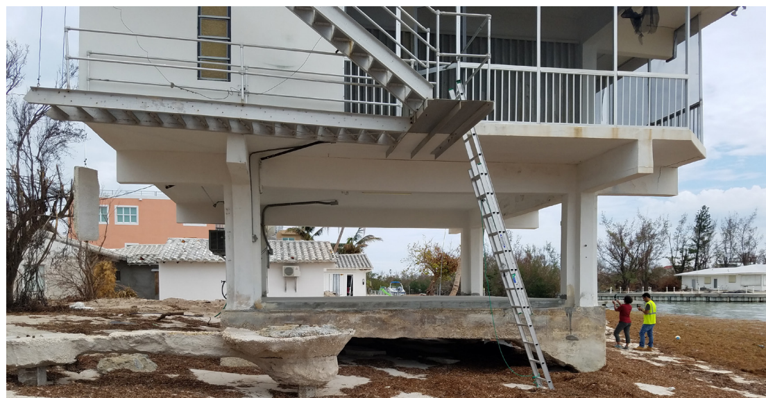
Erosion at a beach house at Sombrero Beach, FL. GEER team members Inthuorn Sasanakul (University of South Carolina) and Luis Arboleda Monsalve (University of Central Florida) on the right. (Photo: Nina Stark)
